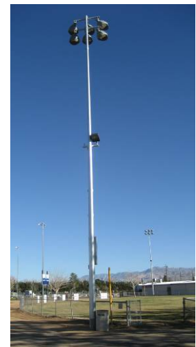
BELOW: the new energy efficient Musco GREEN Structure ballfield lighting system that was installed at James Woody Park, Brewster Park and Mendel Park.
